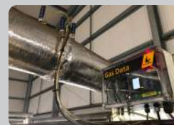
Gas Flow Monitoring
